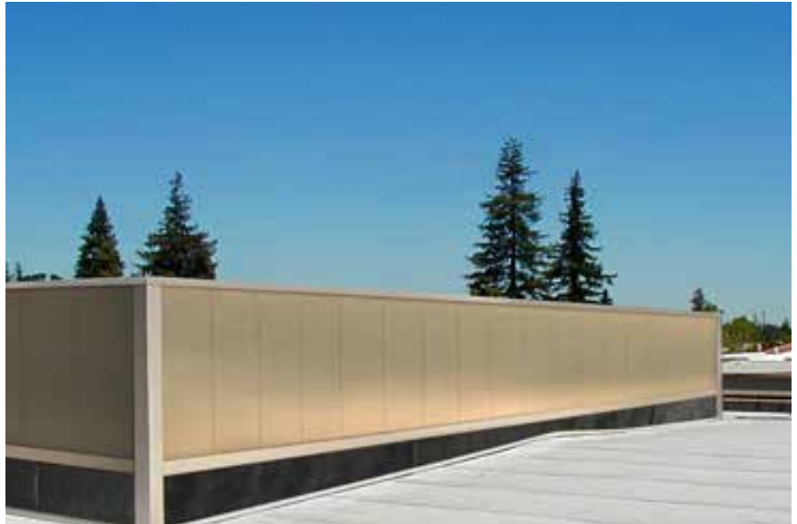
Screened rooftop equipment
